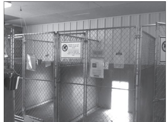
The white vertical sheet metal on the kennel wall is part of the recently completed insulation project.
